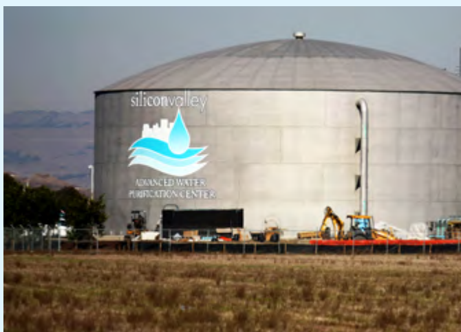
The Santa Clara Valley Water District's Silicon Valley Advanced Water Purification Center in San Jose, CA. Courtesy of Santa Clara Valley Water District.
