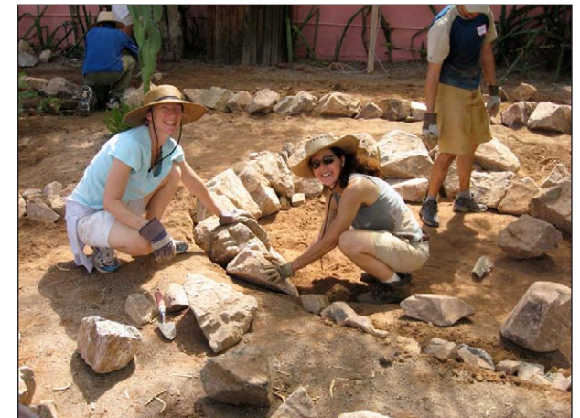
Volunteers pitch in to create bioretention basins at a ROW GI site in Tucson.
