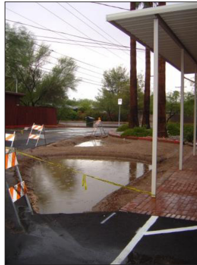
At this Tucson City Council Ward office, asphalt was removed from an unused portion of the parking lot. Runoff from the lot (foreground) and the adjacent building fills the unfinished basins in a summer storm.
