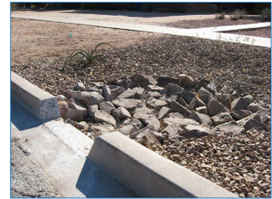
A rock apron protects against soil erosion where curb cuts draw stormwater into bioretention areas.
