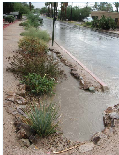
A curb cut draws stormwater from the street into a bioretention basin in the right-of-way.
