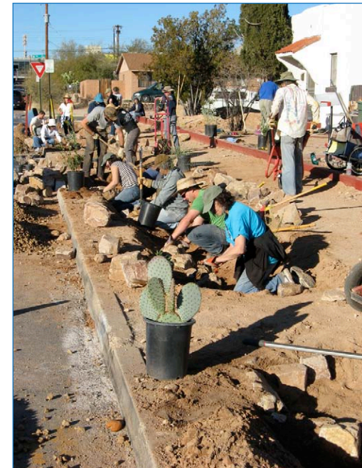
At a WMG-led workshop in Tucson, volunteers install bioretention basins in the right-of-way.
