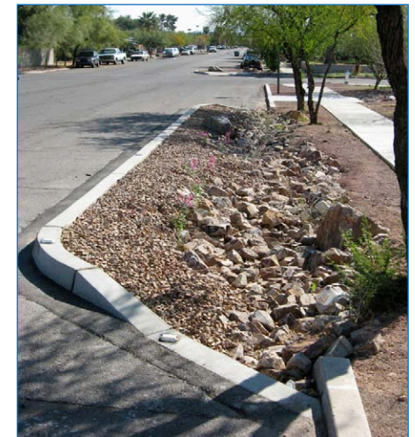
In this just-installed chicane, 4"-8" rock is used in the channel where stormwater will flow rapidly, and 1" gravel covers upslope areas.
