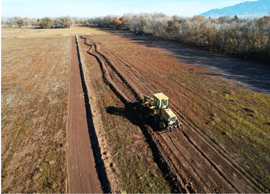
Figure 5. Grading of field 4A in Fall 2023. Top of photo is north direction.
